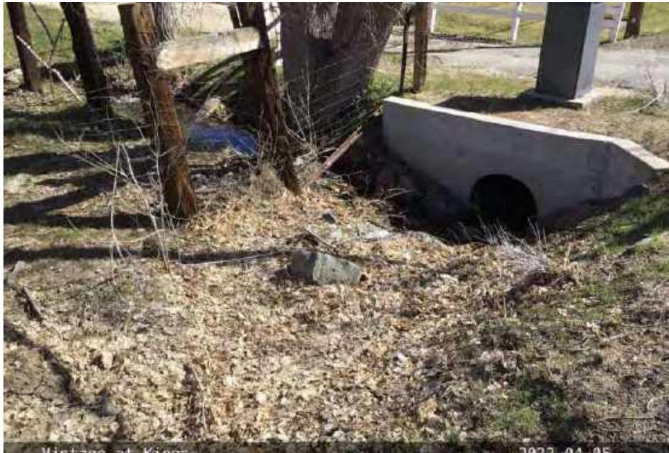
Photo 10. AR-3 at southeast corner of Survey Area where waters, when present, exit off-site into storm drain. View looking northeast.
