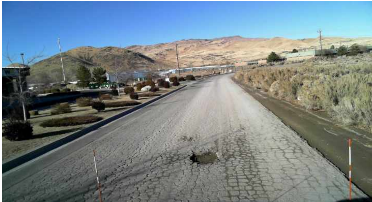
Figure 8. Pavement in Failed condition category (PCI 10-0).
