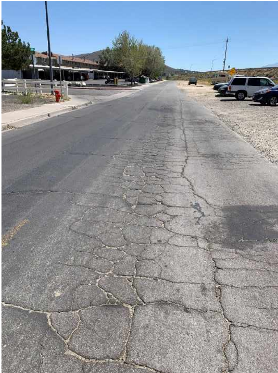
Figure 6. Pavement in Very Poor condition category (PCI 40-26).
