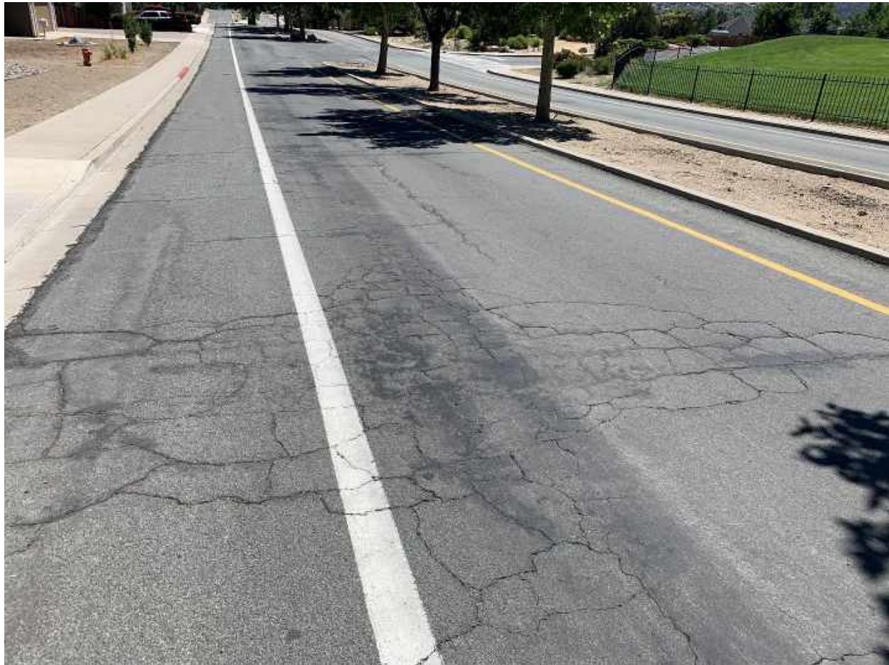
Figure 5. Pavement in Poor condition category (PCI 55-41).
