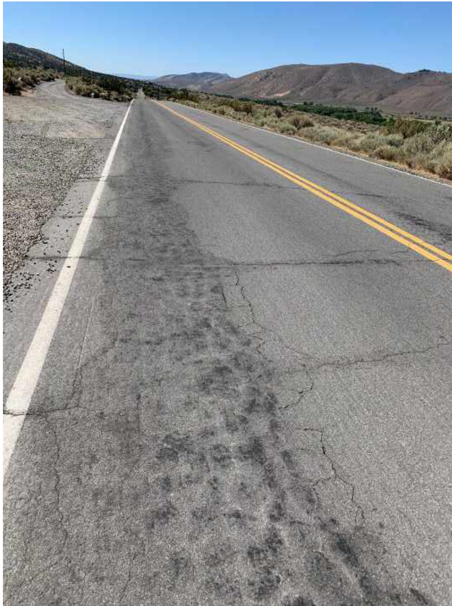
Figure 7. Pavement in Serious condition category (PCI 25-11).
